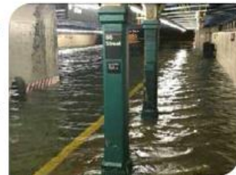
New York City's subway system, the nation's busiest, sustained the worst damage in its 108 years of operation on October 29, 2012, as a result of Hurricane Sandy. Millions of people were left without service for at least a week.
