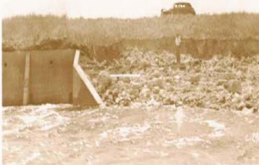
FIG. 2 SERIOUS EROSION ON UNPROTECTED LEVEE FACE
